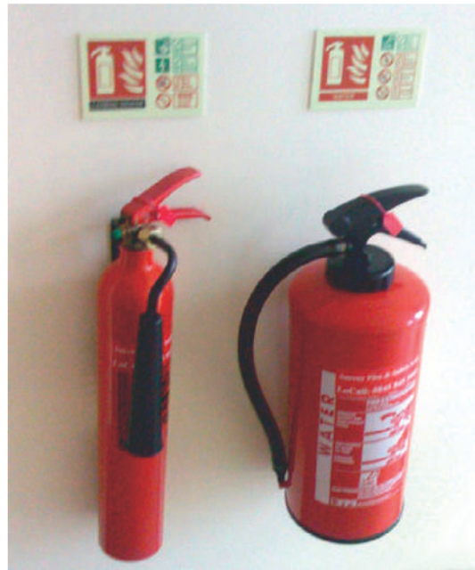
Figure 1.44 CO 2 and water extinguishers and information posters
